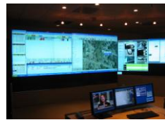
Network Operation Control
